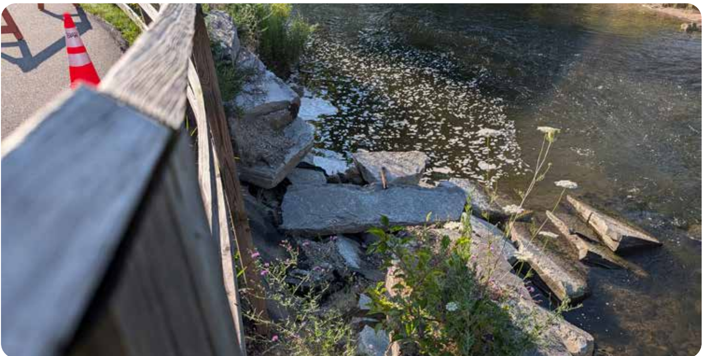
FAILED RETAINING WALL | LOOKING SOUTHEAST
