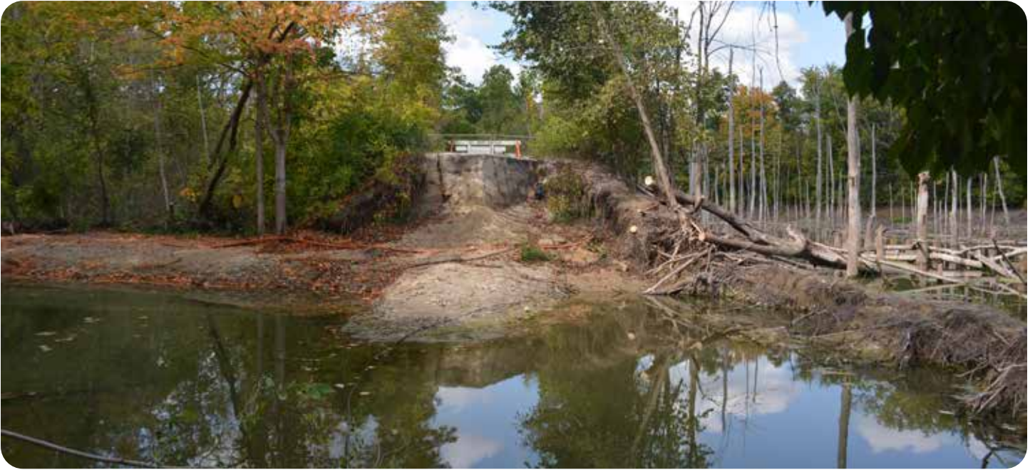
WASHOUT #1 | LOOKING WEST
