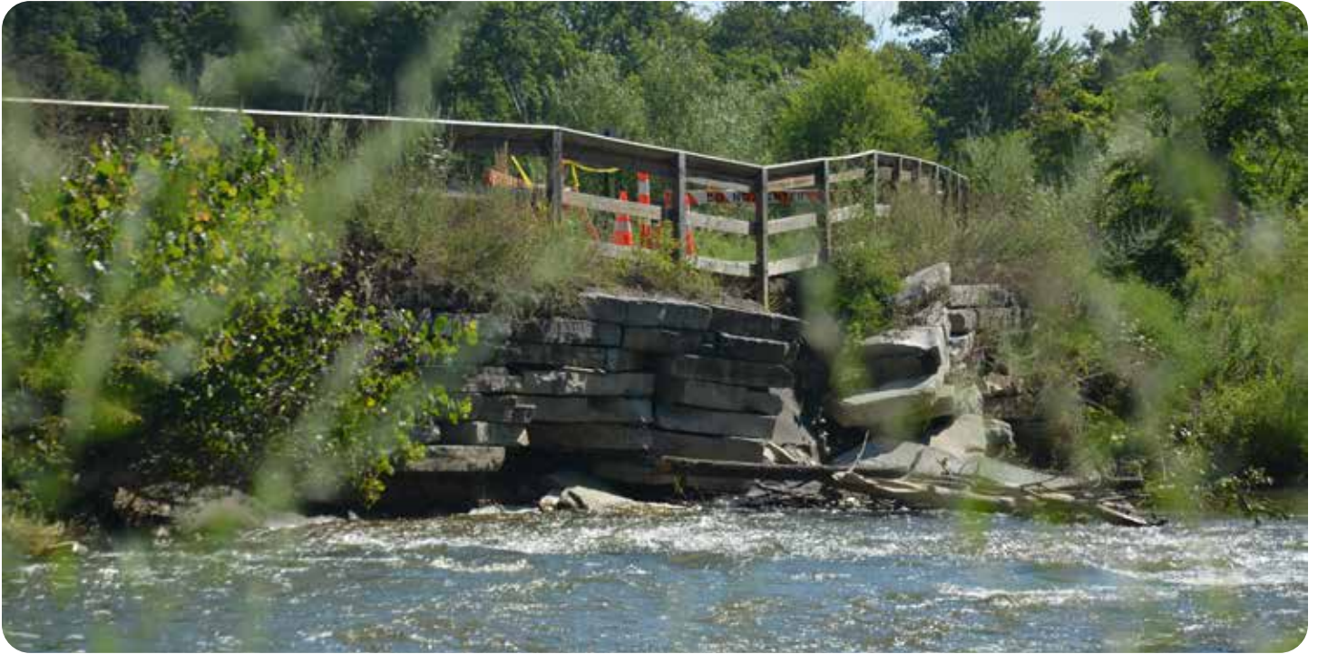
WASHOUT #2 | LOOKING NORTHEAST
